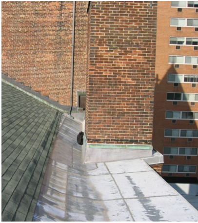
Flat seam lead coated copper gutter comprised of very large pans and suffering from fatigue cracks.
